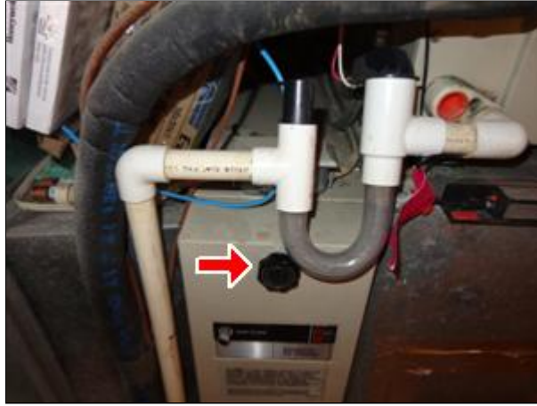
8.0 Picture 2 filter door blocked
