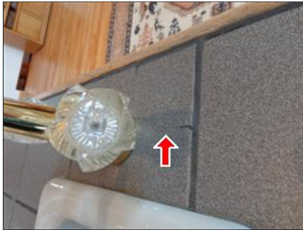
6.6 Picture 1 crack here
