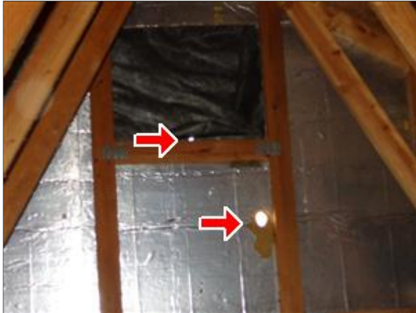
2.0 Picture 4 two holes viewed in attic
