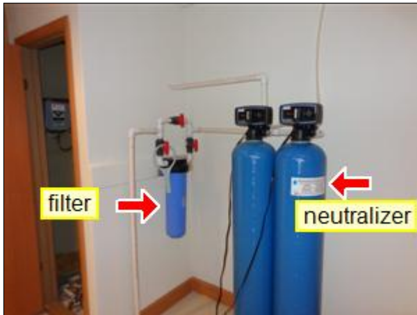
6.0 Picture 1 view of equipment
