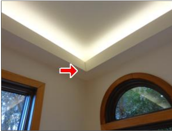
4.0 Picture 1 cracks here
