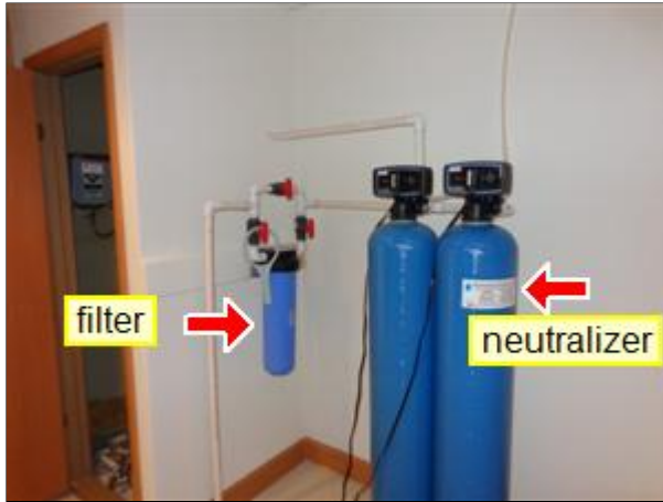
6.0 Picture 1 view of equipment
