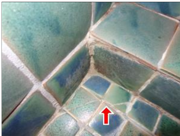
6.6 Picture 6 cracks loose tile
