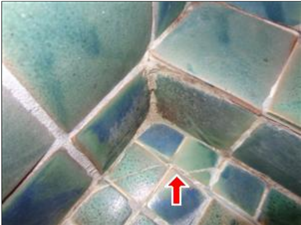
6.6 Picture 6 cracks loose tile
