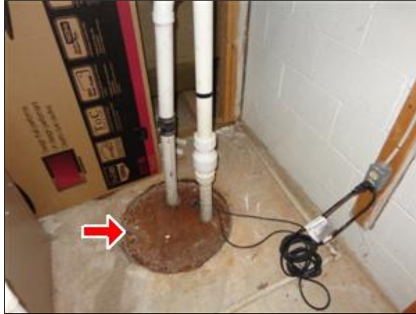
6.7 Picture 1 motor in pit here
