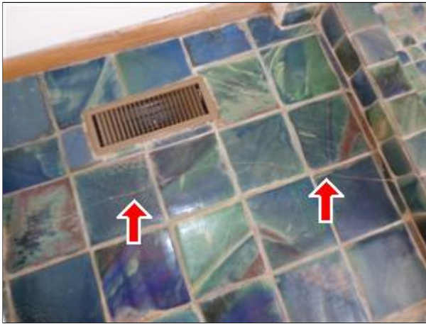
6.6 Picture 2 floor outside shower
