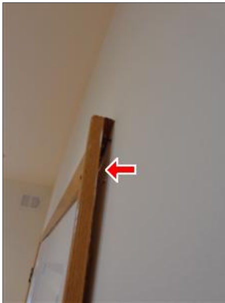
4.5 Picture 2 trim loose
