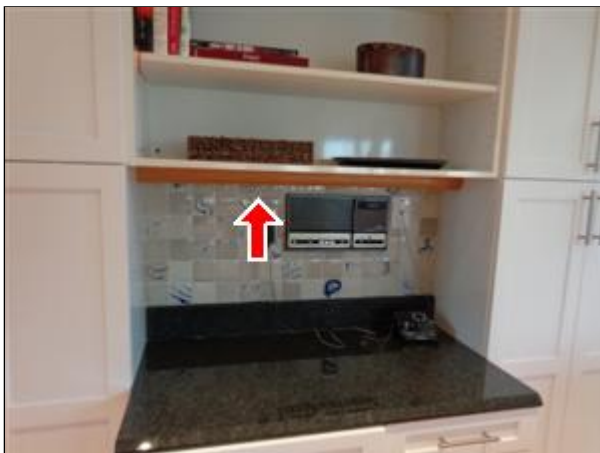
7.3 Picture 4 light not working
