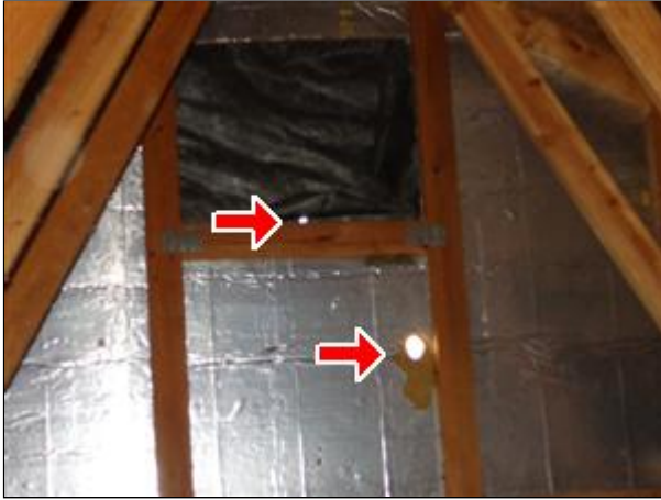
2.0 Picture 4 two holes viewed in attic
