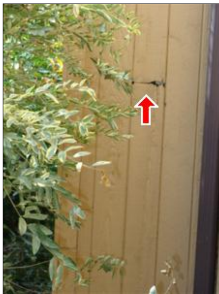
2.0 Picture 3 trim on fireplace left side of home rot
