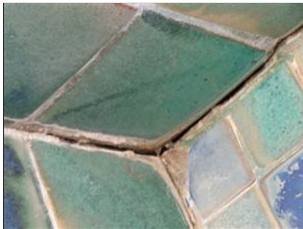
6.6 Picture 8 voids in corner
