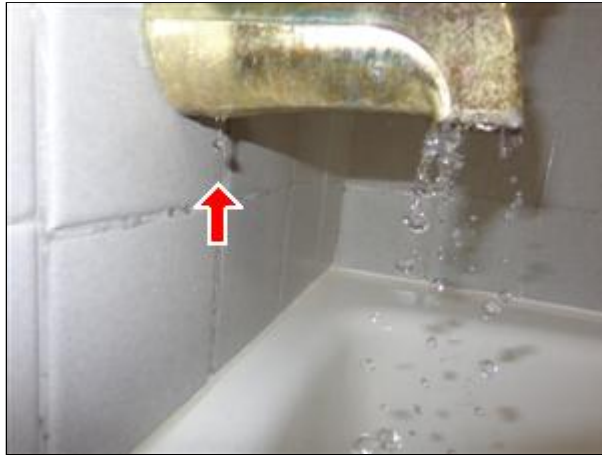
6.0 Picture 6 leaking here
