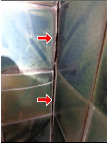
6.6 Picture 5 large void in corner
