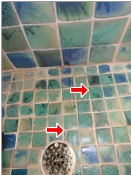
6.6 Picture 4 crack here
