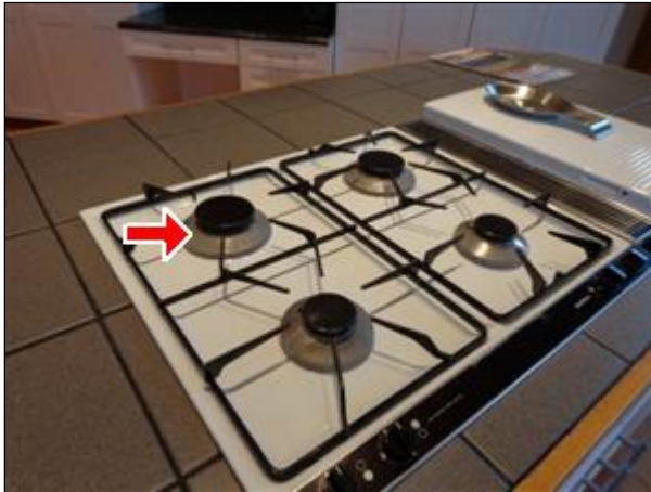
10.1 Picture 1 not lighting
