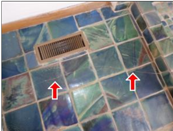
6.6 Picture 2 floor outside shower
