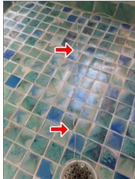
6.6 Picture 3 crack in shower
