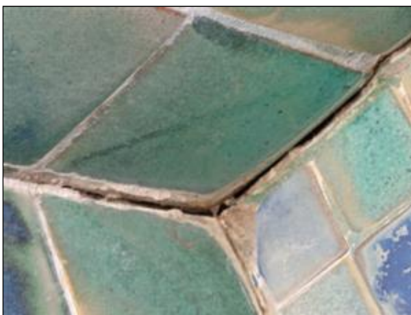
6.6 Picture 8 voids in corner
