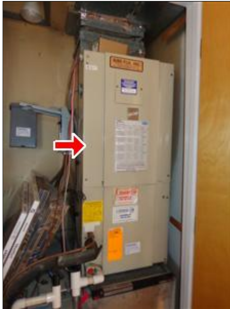
6.7 Picture 2 no overflow pan only safety on trap
