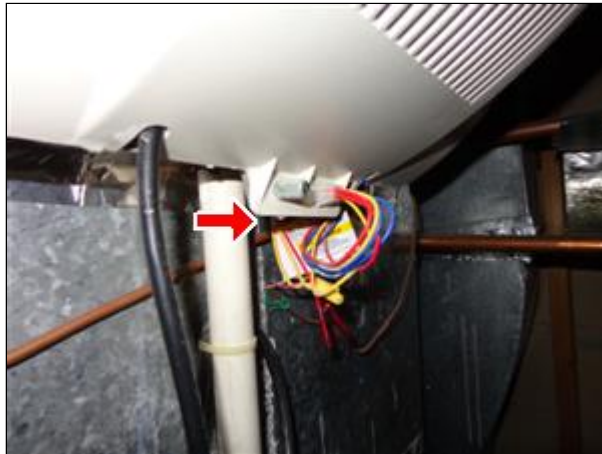
8.1 Picture 4 leaking here
