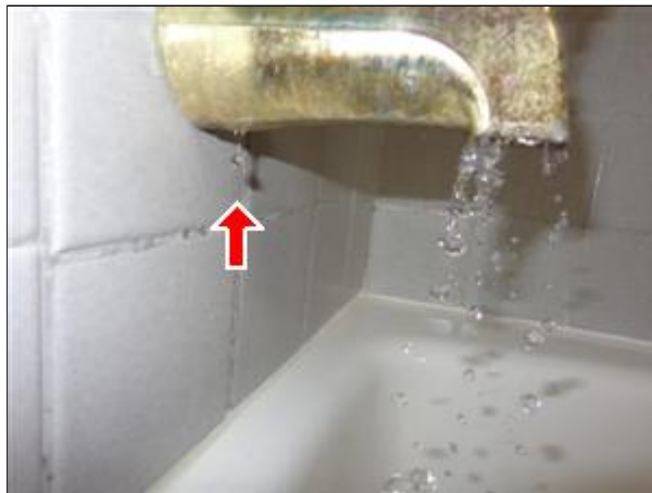
6.0 Picture 6 leaking here
