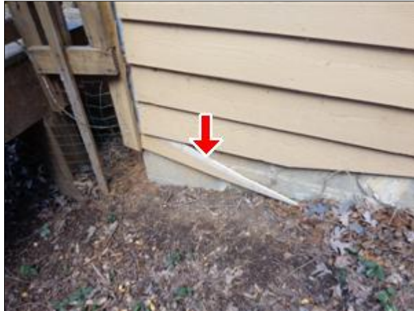
2.0 Picture 10 loose siding
