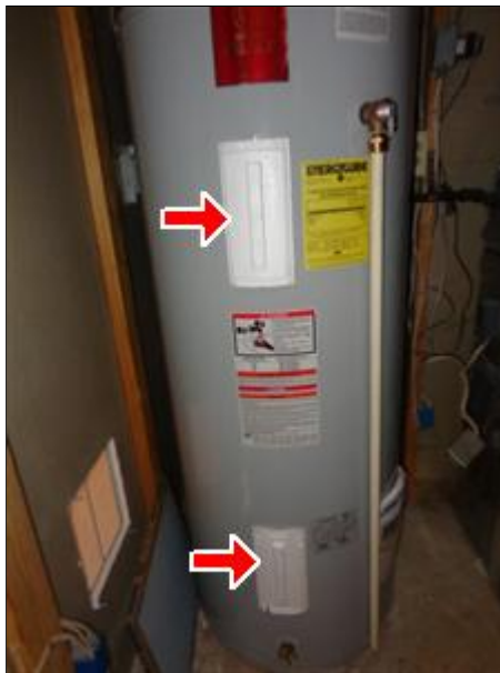
6.1 Picture 1 covers go here and are on top of heater
