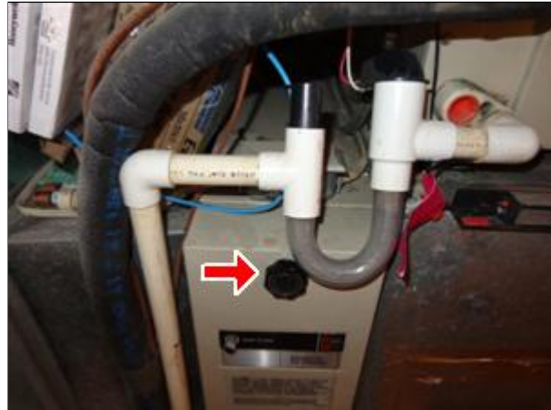
8.0 Picture 2 filter door blocked
