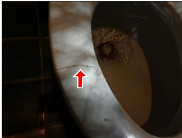
6.0 Picture 5 cracked seat
