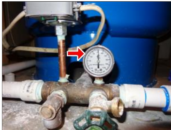
6.0 Picture 3 water in gauge
