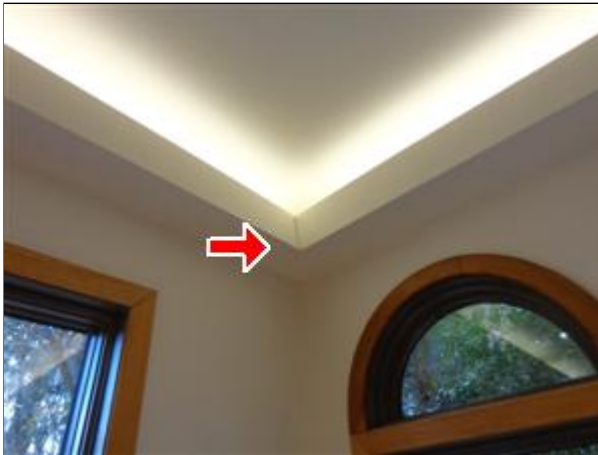
4.0 Picture 1 cracks here
