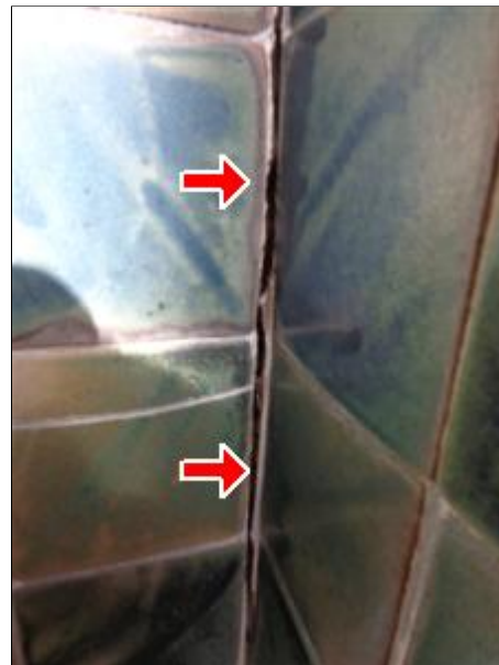
6.6 Picture 5 large void in corner
