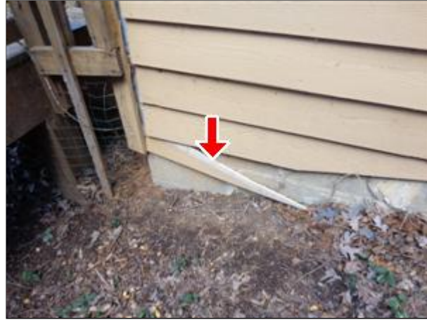
2.0 Picture 10 loose siding
