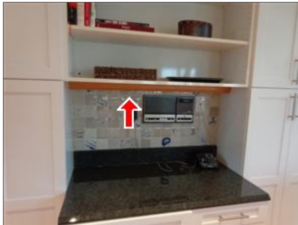
7.3 Picture 4 light not working
