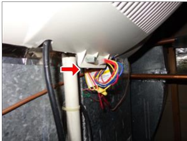
8.1 Picture 4 leaking here
