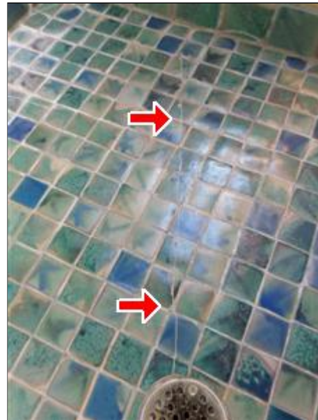
6.6 Picture 3 crack in shower
