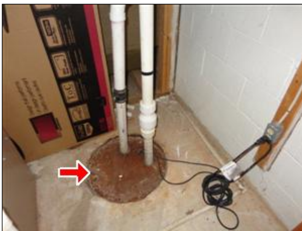
6.7 Picture 1 motor in pit here
