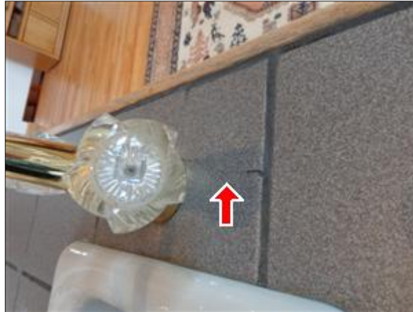
6.6 Picture 1 crack here
